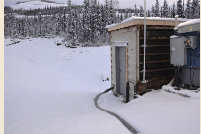
DG4 Sump, October 2025
