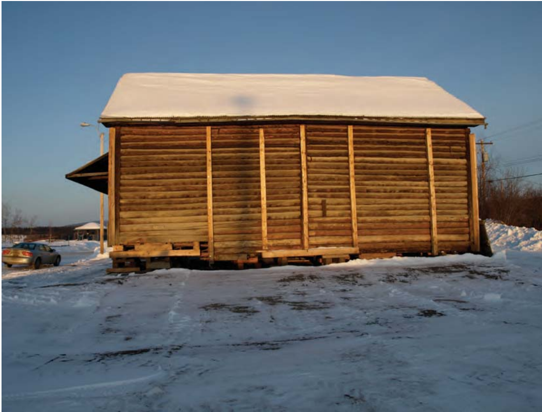
7. east wall: the building is supported with a series of strongbacks. The one in the middle of the wall is located on the mid wall vertical log
