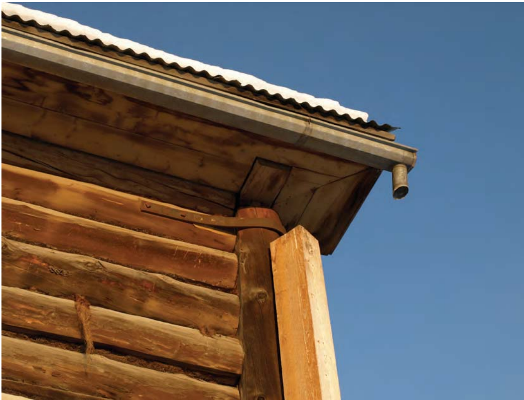
8. east wall, detail of upper rear corner, showing the typical steel strap and galvanized gutter. The squared log which is fitted into the soffit shows clearly
