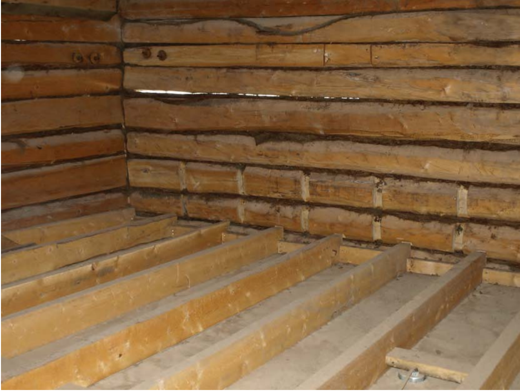
32. area above false ceiling: regularly spaced notches show on the walls, suggesting upper floor framing consistent with the 1 1/2 storey wall heights. The existing construction consists of full dimension 2x6 framing @ 16 o.c., supported at mid span by the "truss"
