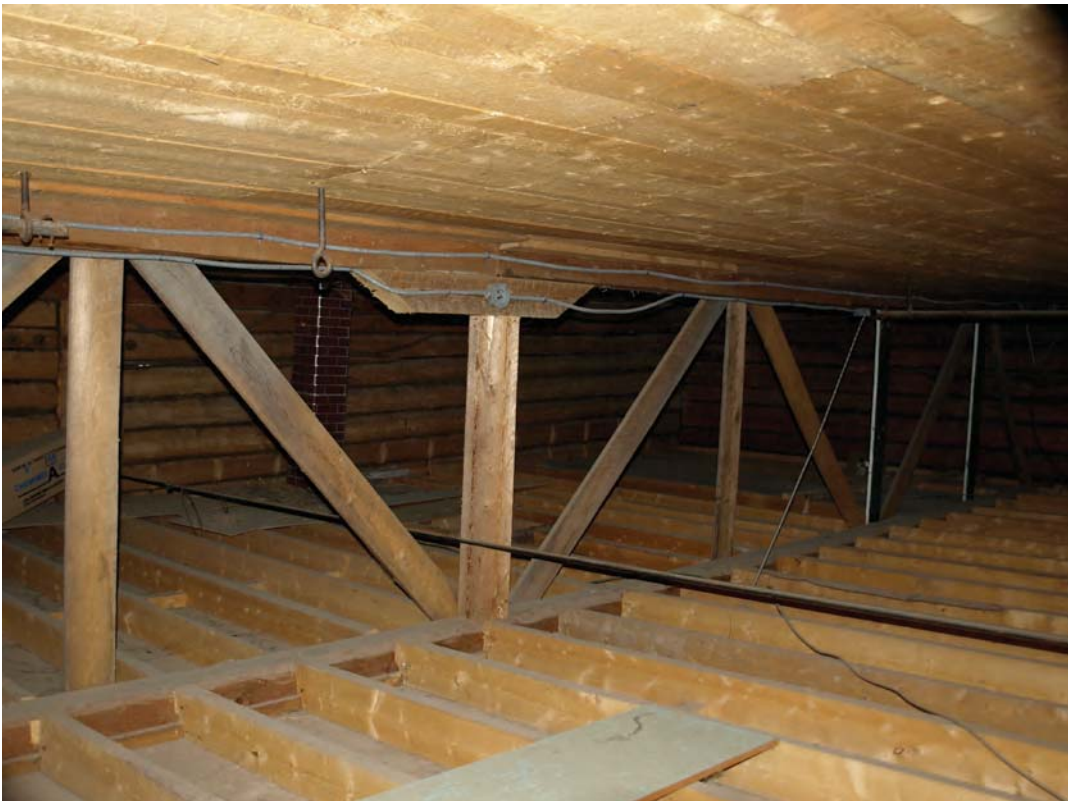
33. area above false ceiling, the truss: the lower ceiling joists are notched out at the truss for a 1x2 ledger. The steel tension rod holding the central posts shows in the middle of the photograph
