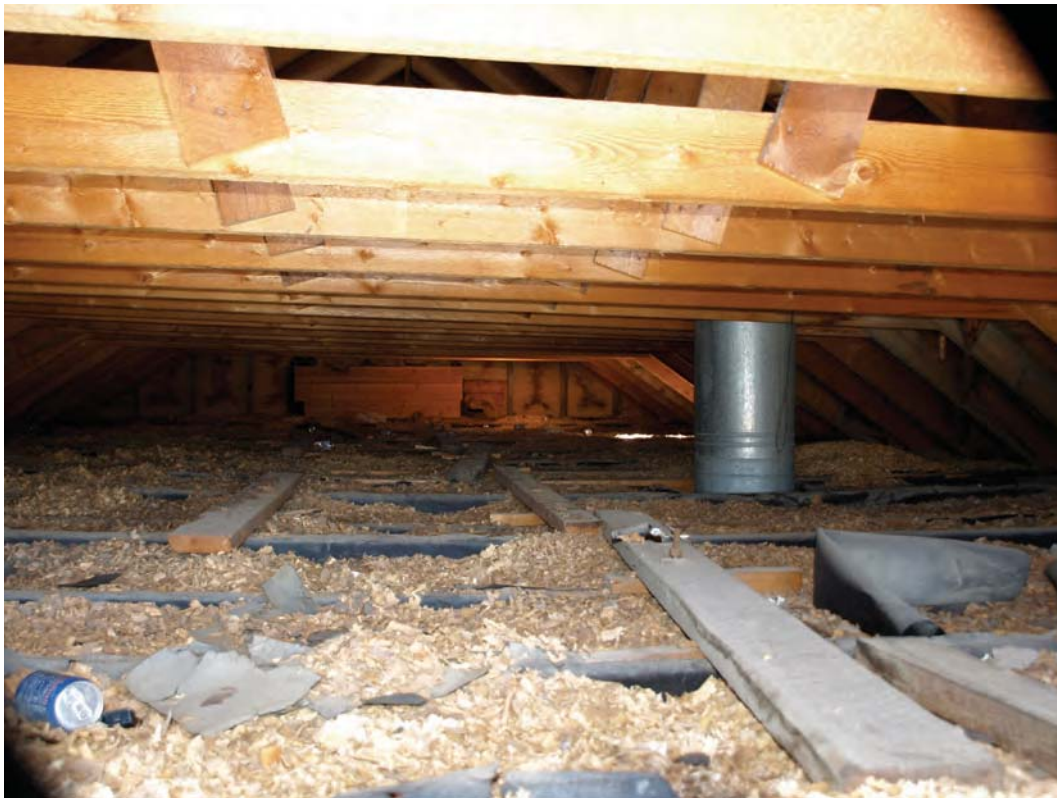
31. attic: the cross ties show in the upper part of the photograph, the ceiling rafters are below. The space between the rafters is filled with wood chips as insulation. The boards lying on the rafters are through bolted to the pipe hangers which extend through the ceiling below (see photos 35 and 36) The chimney flue is in its original location.
