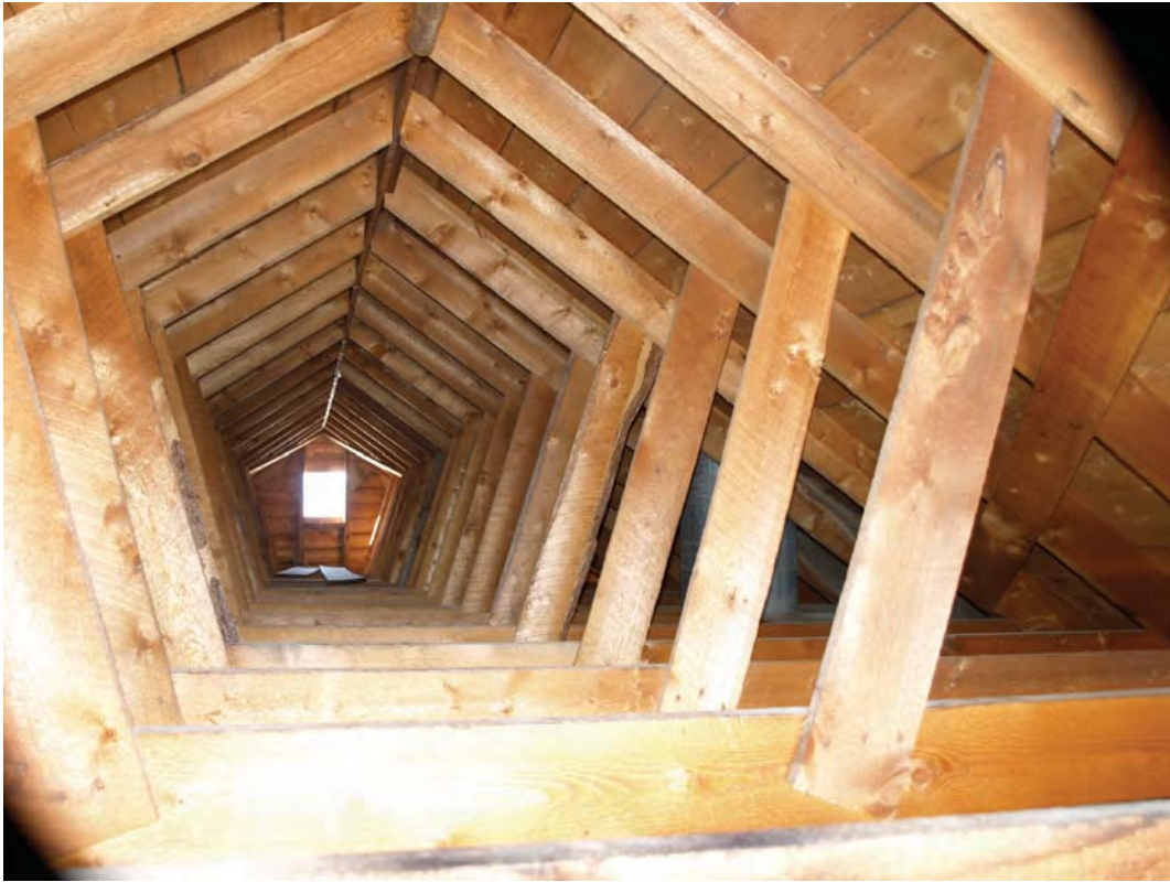
30. attic: the roof is well constructed from full dimension lumber. 1x6 struts connect the rafters to the mid level cross ties
